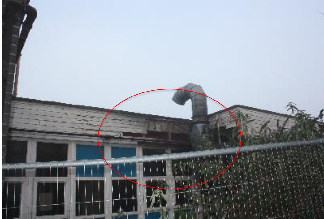
Plate 9: An image showing the east elevation of the building (Hotspot Area 3, is indicated by the red circle)
