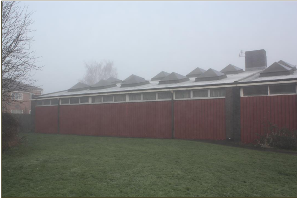
Plate 5: Another image of the southern elevation of the building to be demolished.
